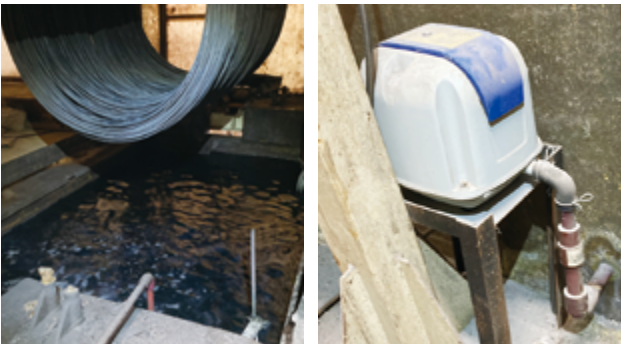
Sulfuric acid tank in pickling line and a newly introduced blower
