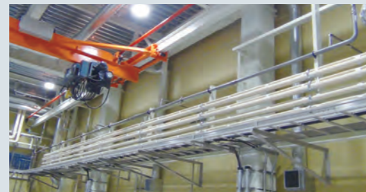
FP35 installed, at M Building of Sango's Toyota Technical Center
